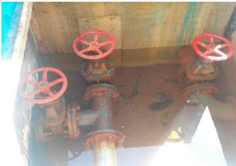
Pipa pengontrolan air
